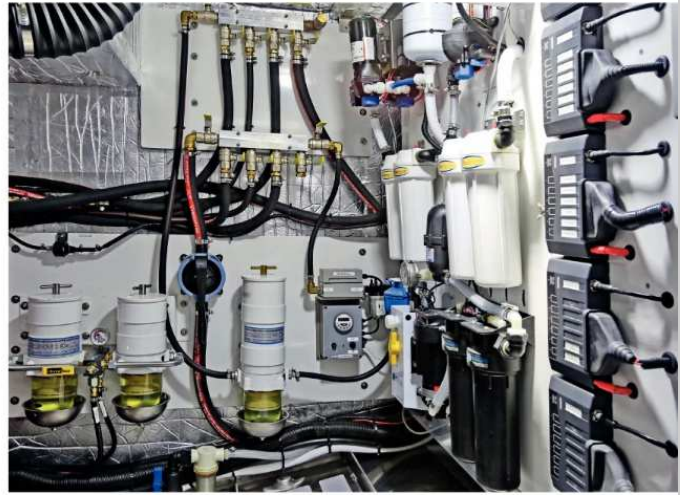
The spacious engineroom allows easy access to filters, fuel management, fresh water filters and switch panels to over-ride CZone.
